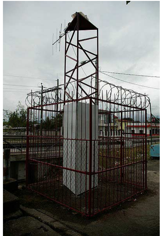
Fig. 5. 5 Meter Antenna Tower with Security
